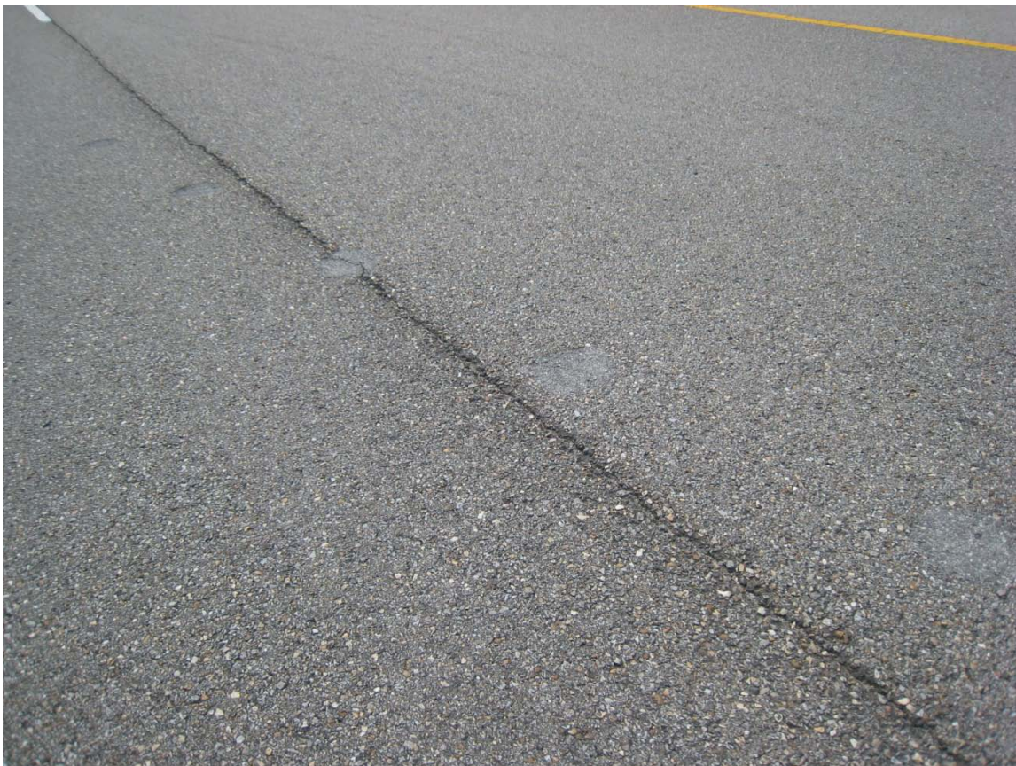
FIGURE 24 Site #3 Approximately Two Years After Construction.
