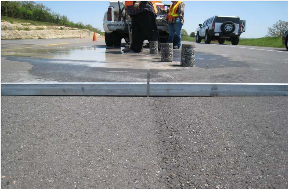
FIGURE 5 Site #3 – Fair/Poor Condition.
