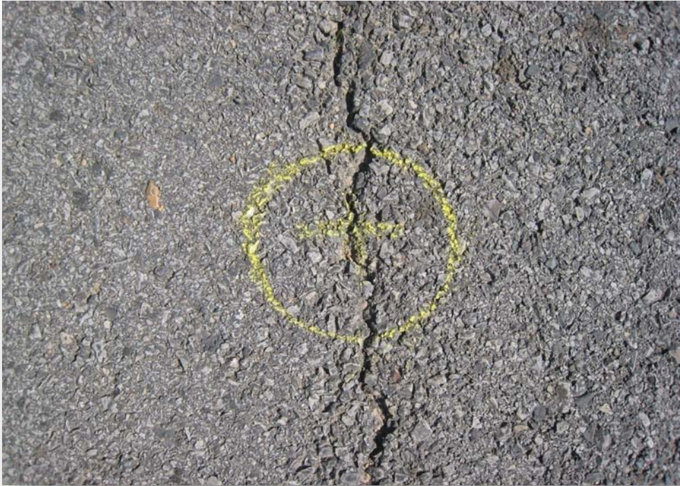
FIGURE 4 Site #2 – Fair/Poor Condition.
